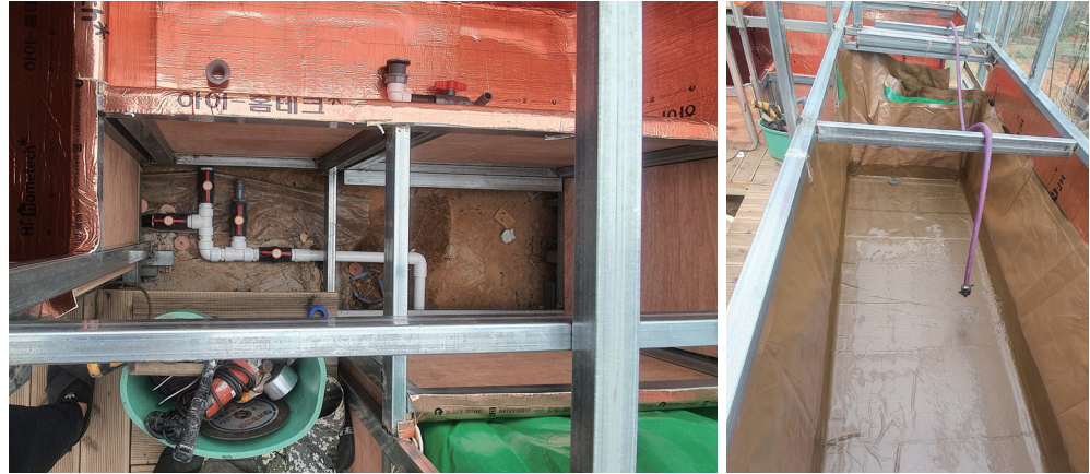
Pipes connecting the fish tanks to the purification tank
