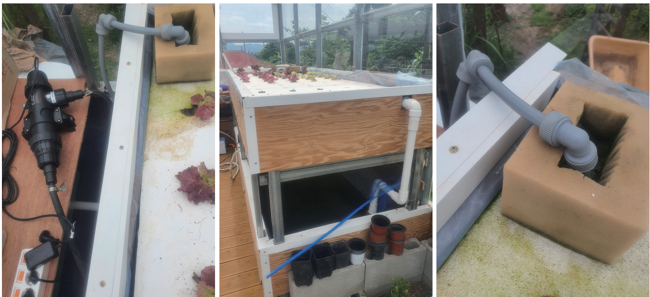
Motor pump pumping water from purification tank to grow bed
